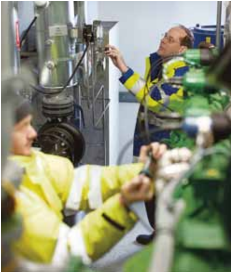
> Siemens plant Krefeld
